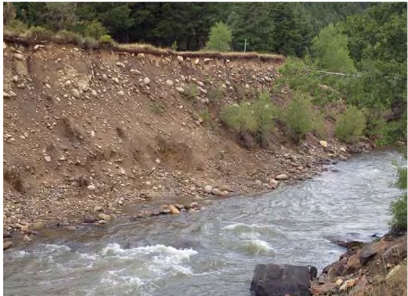
Channel bank erosion on this barren bank along I-70 is clearly evident in this reach of Clear Creek upstream of Idaho Springs.
