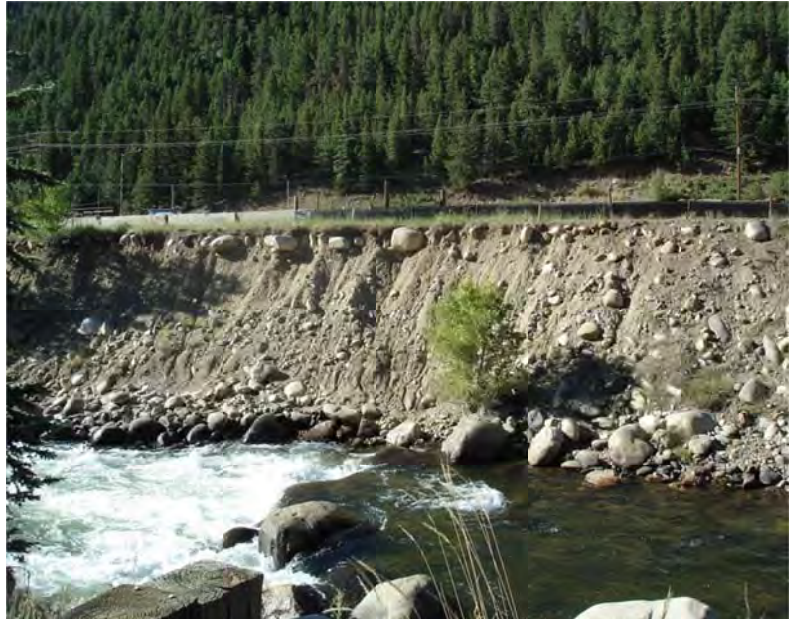
This Clear Creek channel bank adjacent to I-70 is not stable and is actively eroding, especially during periods of high flow.
